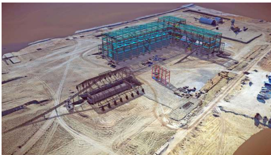
AAEngineering was tasked with overall design, procurement, and construction works that required upgrading existing energy and mining infrastructure. Image courtesy of AAEngineering Group.
