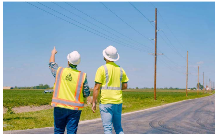
Despite having to respot, respan, and realign the design due to supply constraints, PLS-CADD helped the design team create an initial design for bidding just one day after the storm.
